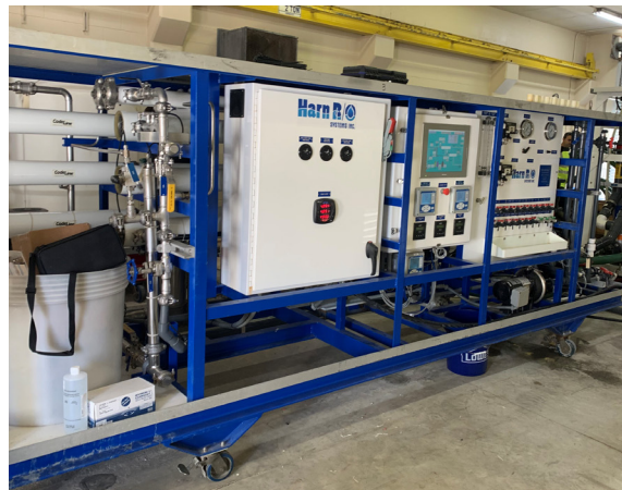
Reverse Osmosis at Plant City's Demonstration Facility
