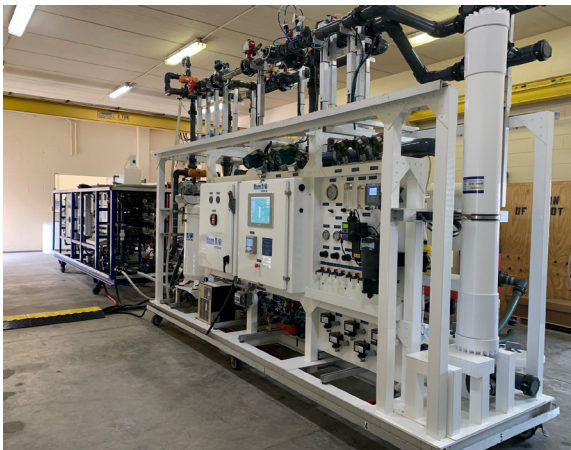
Membrane Filtration at Plant City's Demonstration Facility
