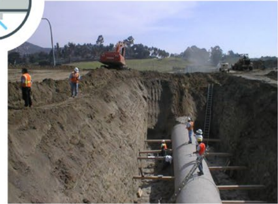
Crossover Pipeline San Diego County Water Authority
