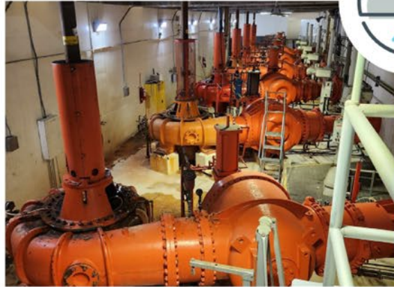
Pump Station 2 City of San Diego
