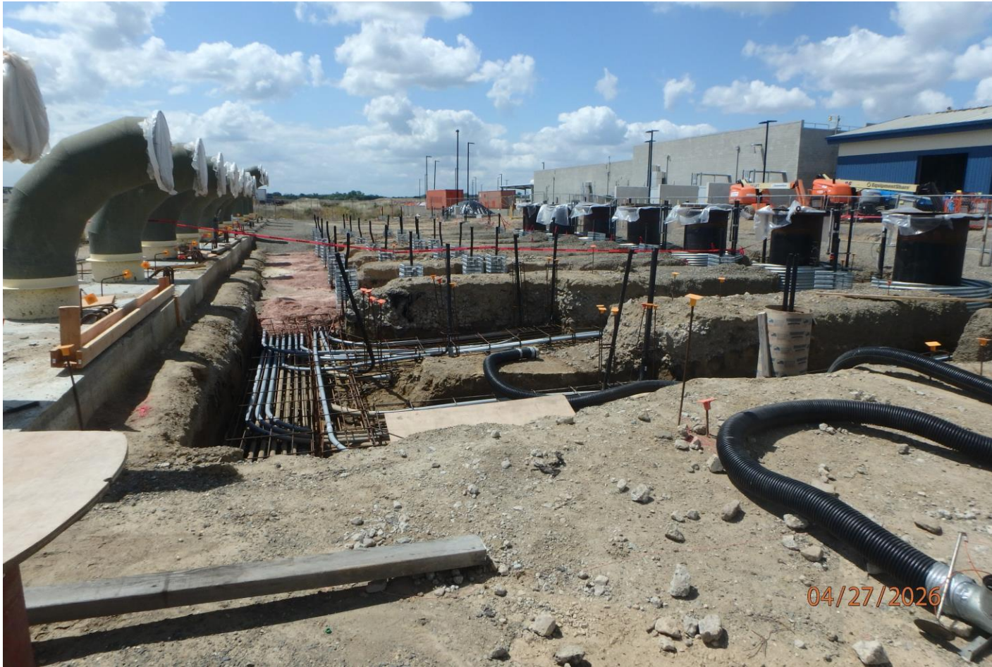
Installed Pump Cans, Duct Banks, and Discharge Elbows
