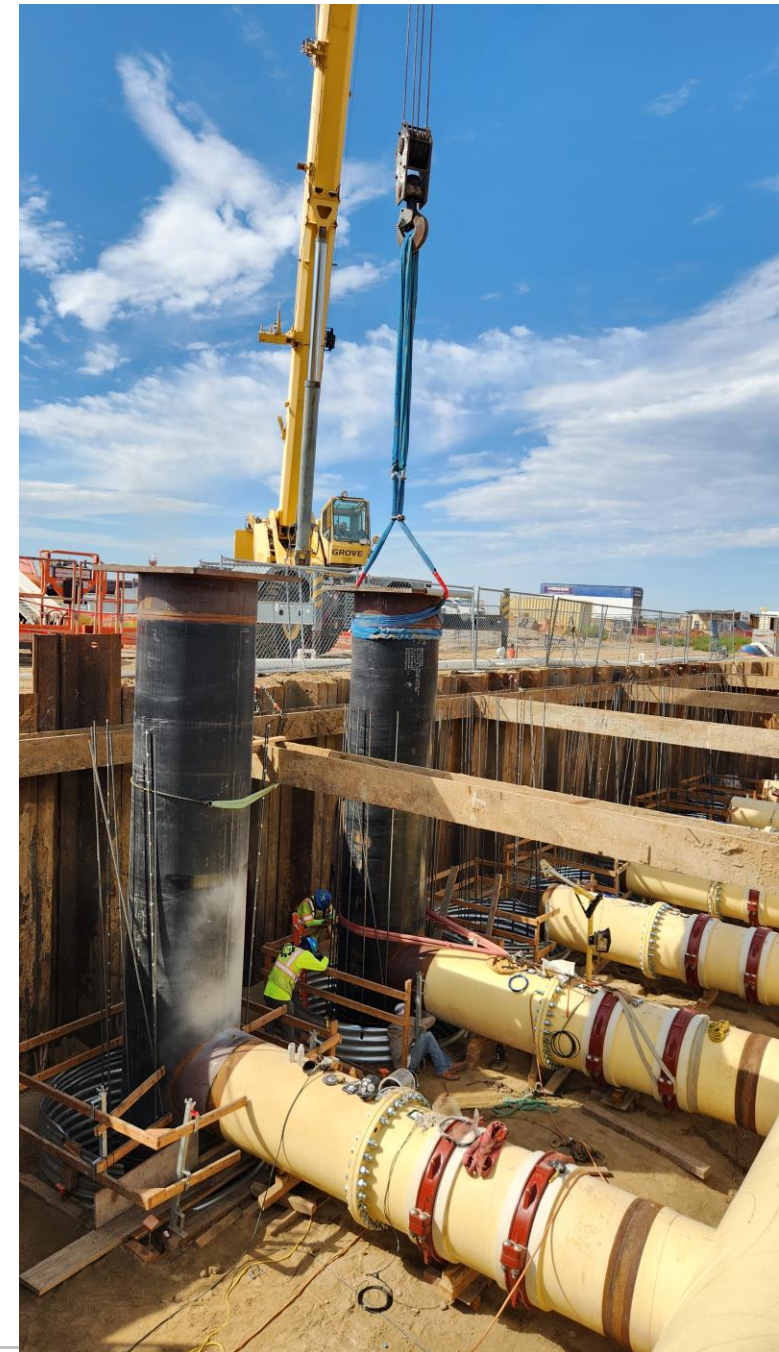
Suction Side - Vertical Turbine Pump Can Installation
