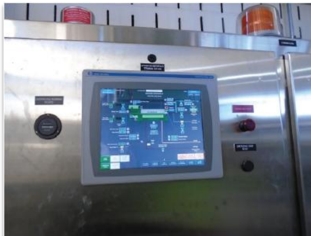
FIGURE 11.3: Typical local operator interface [WWTF 3 Ch13 p10 Figure13.7]
