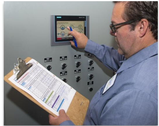
FIGURE 12.1: Operator SOPs should be maintained and followed to ensure consistent actions by staff [Photo credit: San Francisco Public Utilities Commission. Permission to use.]
