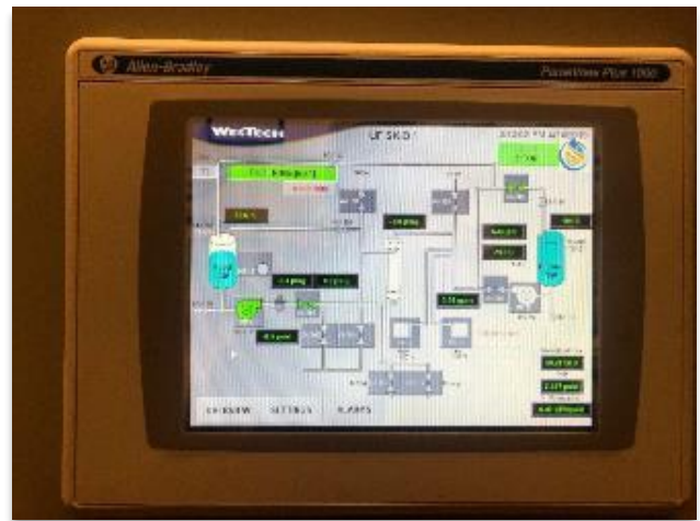
FIGURE 11.2: Operators use process control systems to access information on the treatment system in real time [Photo credit: San Francisco Public Utilities Commission. Permission to use.]
