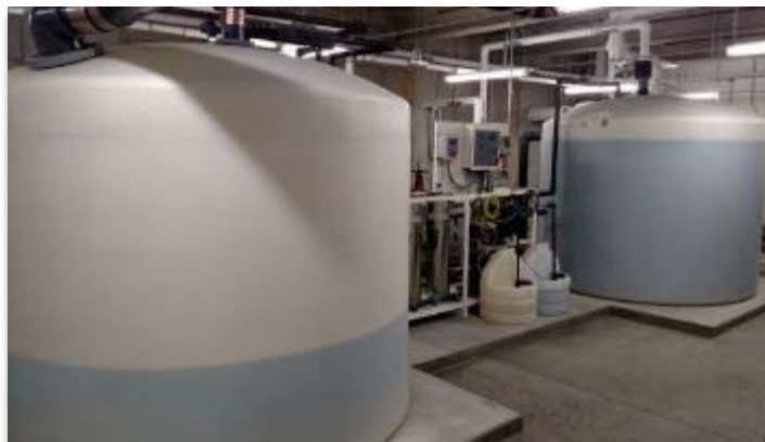
FIGURE 13.2: Tanks used for storing water in an ONWS [Photo credit: Cathy Dacanay, Chemsearch Fe]
