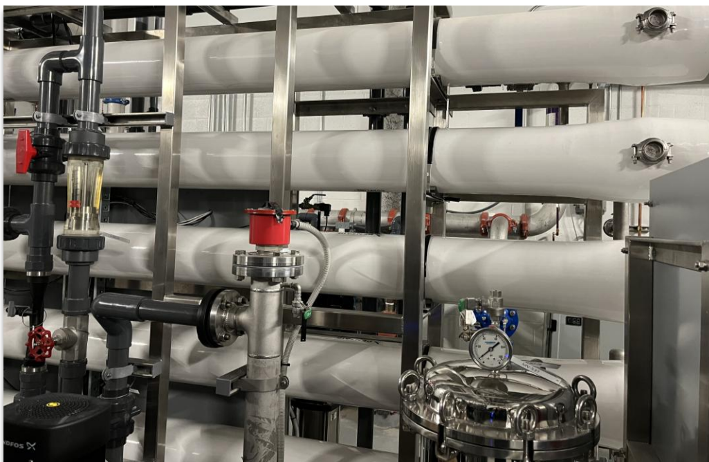
A reverse osmosis system is being used to treat blackwater at Mission Rock in San Francisco, CA [Photo credit: San Francisco Public Utilities Commission. Permission to use.]
