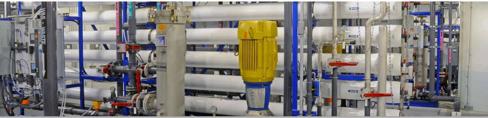
Onsite reuse system's mechanical room at Philip Morris USA in Richmond, VA [Photo credit: Sustainable Water]
