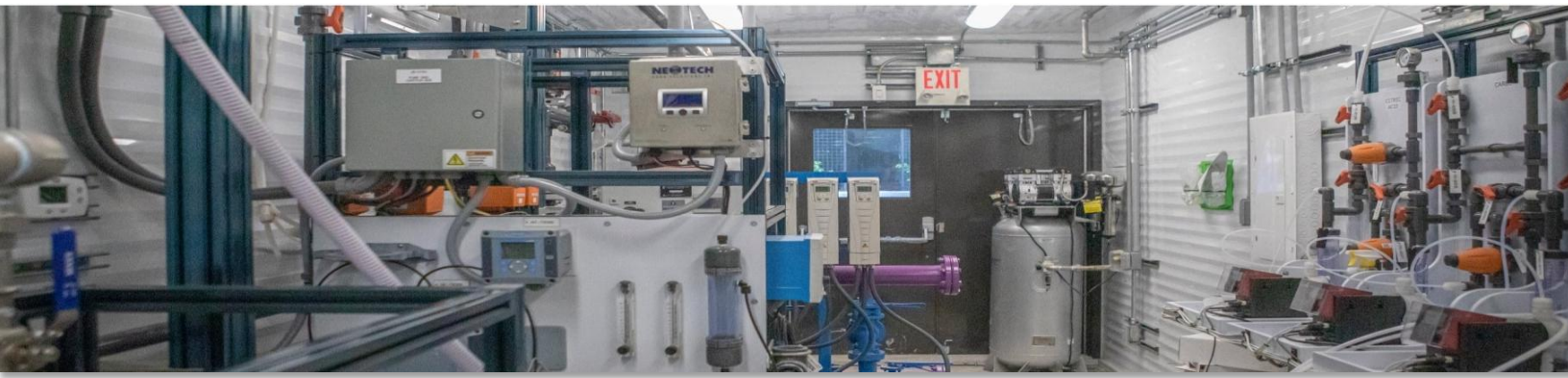
Onsite water reuse treatment system [Photo credit: Austin Water]
