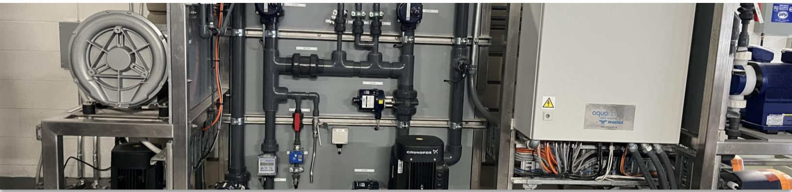
MBR system at Mission Rock in San Francisco, CA [Photo credit: San Francisco Public Utilities Commission]
