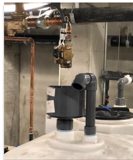
FIGURE 13.3: Example of an air gap protecting the potable water supply from potential backflow [Photo credit: San Francisco Public Utilities Commission. Permission to use.]
