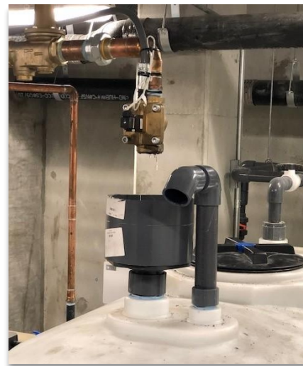
FIGURE 13.3: Example of an air gap protecting the potable water supply from potential backflow [Photo credit: San Francisco Public Utilities Commission. Permission to use.]
