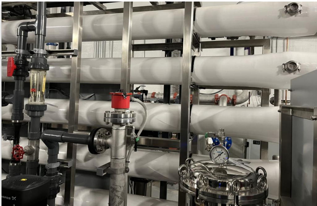
A reverse osmosis system is being used to treat blackwater at Mission Rock in San Francisco, CA [Photo credit: San Francisco Public Utilities Commission. Permission to use.]
