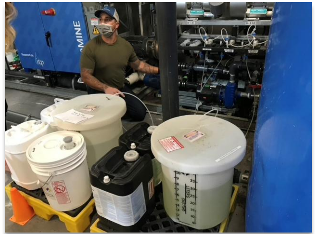
FIGURE 8.3: A combined graywater and rainwater treatment system at 1550 Mission in San Francisco, California, uses chlorine to maintain a disinfectant residual to provide protection against opportunistic pathogens such as Legionella [Photo credit: San Francisco Public Utilities Commission]
