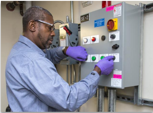
FIGURE 3.1: Operator performing start-up testing [Photo credit: San Francisco Public Utilities Commission]
