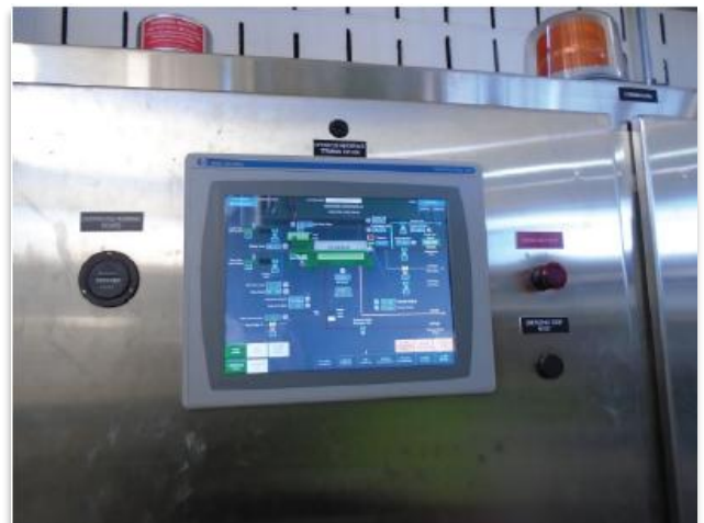
FIGURE 11.3: Typical local operator interface [WWTF 3 Ch13 p10 Figure13.7]
