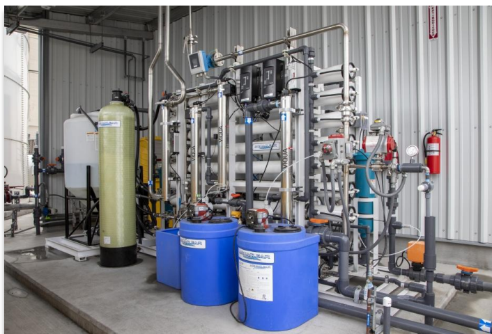
FIGURE 10.2: Blue tanks store liquid chemicals for use in an ONWS [Photo credit: San Francisco Public Utilities Commission. Permission to use.]
