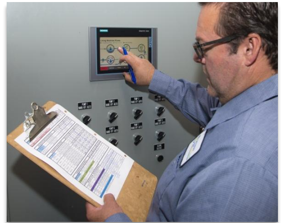
FIGURE 12.1: Operator SOPs should be maintained and followed to ensure consistent actions by staff [Photo credit: San Francisco Public Utilities Commission. Permission to use.]
