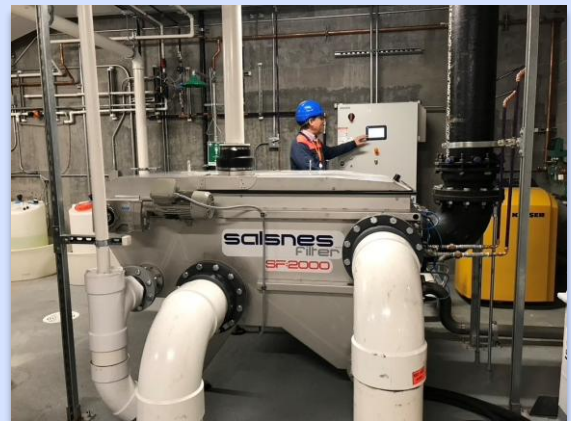
FIGURE 5.2: Example of a solids separation filter used at the Salesforce Tower in San Francisco, CA where the building is recycling its blackwater [Photo credit: San Francisco Public Utilities Commission]
