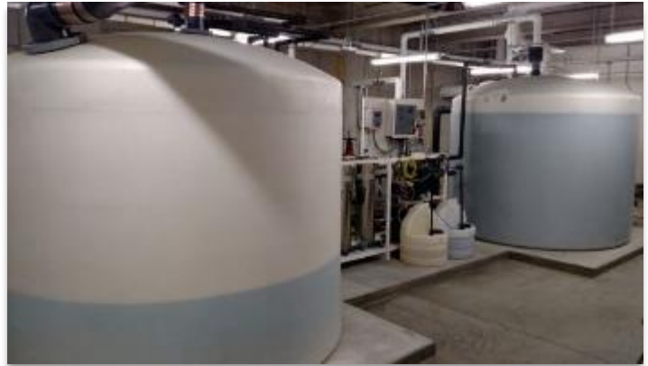
FIGURE 13.2: Tanks used for storing water in an ONWS [Photo credit: Cathy Dacanay, Chemsearch Fe]
