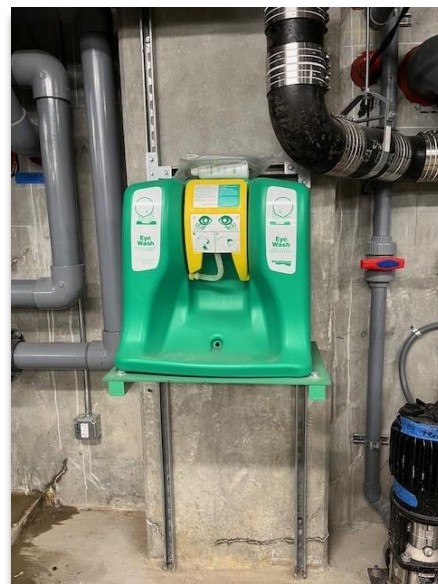
FIGURE 10.1: Example of an eyewash station [Photo credit: San Francisco Public Utilities Commission. Permission to use.]
