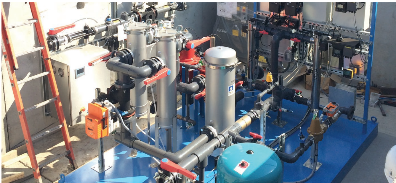
Allianz Field at Midway Development District in Saint Paul, Minnesota has a district-scale rainwater system. Photo credit: City of Saint Paul
