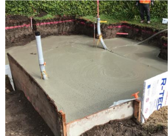
PG&E Metering Pad
