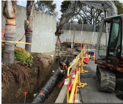
Source Water Pipe
