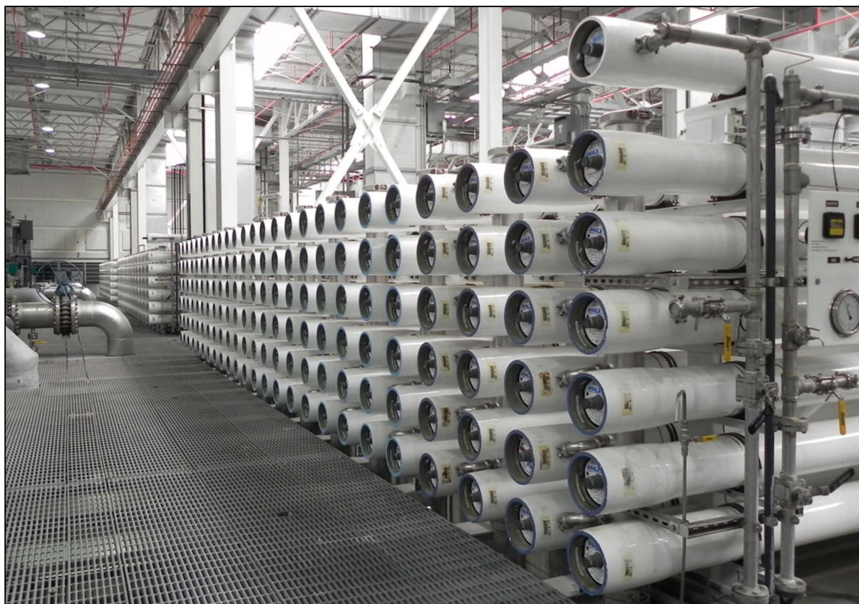
Figure 6 Reverse Osmosis at the Groundwater Replenishment System
