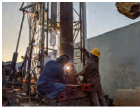
Seawater Intrusion and Prevention Wells and Monitoring Wells Construction in Capitola and Aptos
