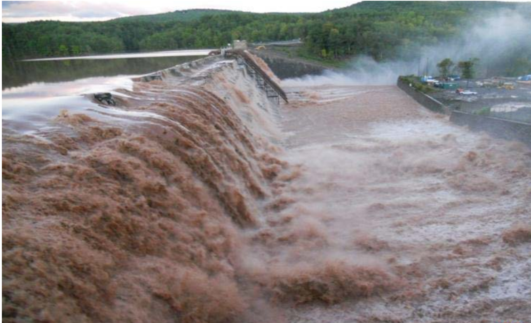
August 2011: Water spills over the Gilboa Dam following Tropical Storm Irene, Gilboa, NY
