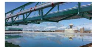
Wichita Falls’ DPR Project went online July 9, 2014 following extensive testing by the City of Wichita Falls and the Texas Commission on Environmental Quality (TCEQ). Shown here is one of their clarifiers.
