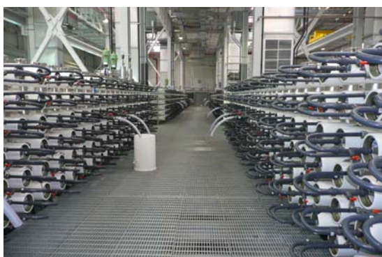
Figure 3.10. OCWD’s RO membrane gallery.
