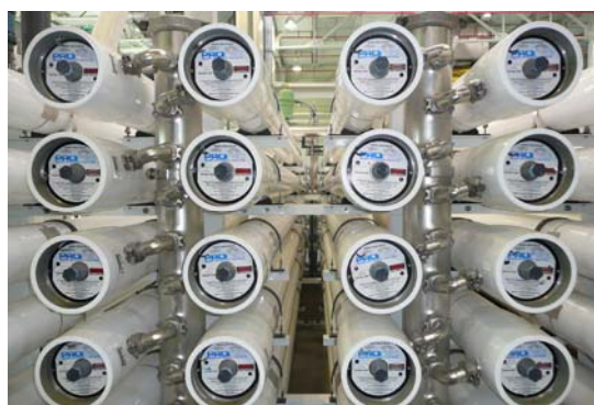
Figure 3.11. OCWD’s RO membrane elements within pressure vessels.
