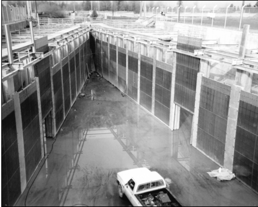
Figure 3.21. Angled screen diversion system at White River.
