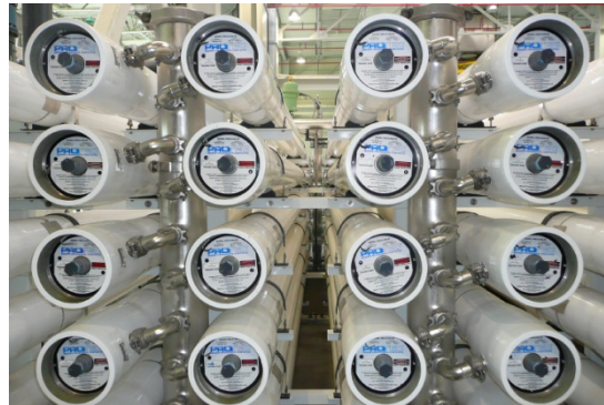
Figure 2.30. OCWD's RO membrane elements within pressure vessels.
