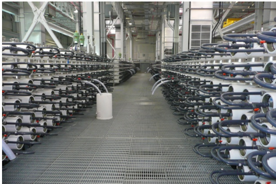
Figure 2.29. OCWD's RO membrane gallery.
