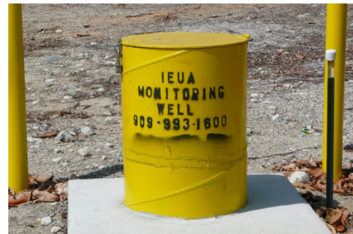
Figure 2.21. 8th St. Basin's perimeter monitoring well.
