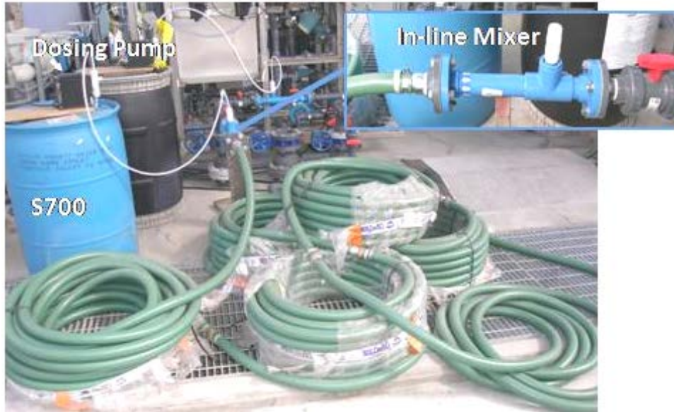
Figure 4.19. S700 coagulant dosing apparatus with 550 ft of 1.5-in. J series hose upstream of the MF pilot unit to simulate 5.3 min of contact time.
